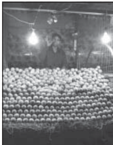
A typical example of unsafe wires for lighting stalls through illegal connections
